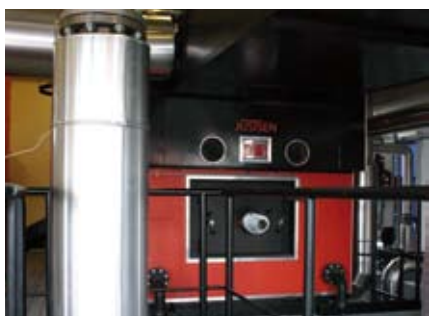
Top part of biomass boiler.
