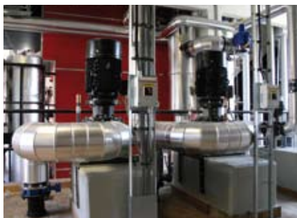
Demand controlled hot water distribution pumps.
